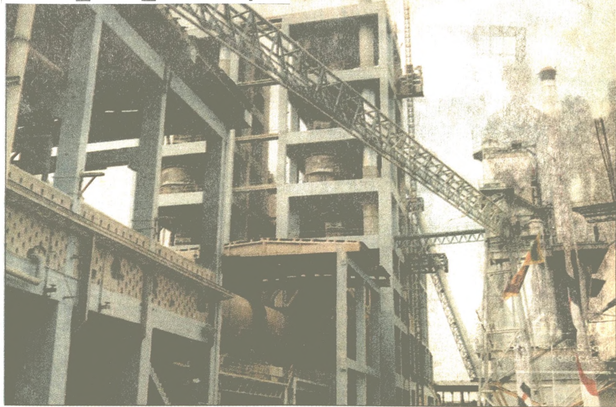
The new 'coal grinding plant'
