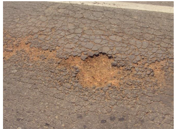
Figure 1 - Distresses observed on the B424 Road
